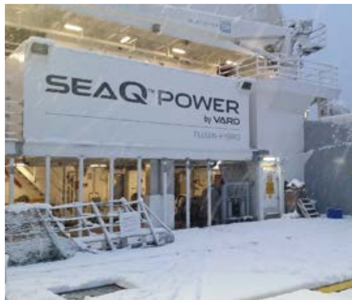
Photo above provided by Vard Electro Canada
